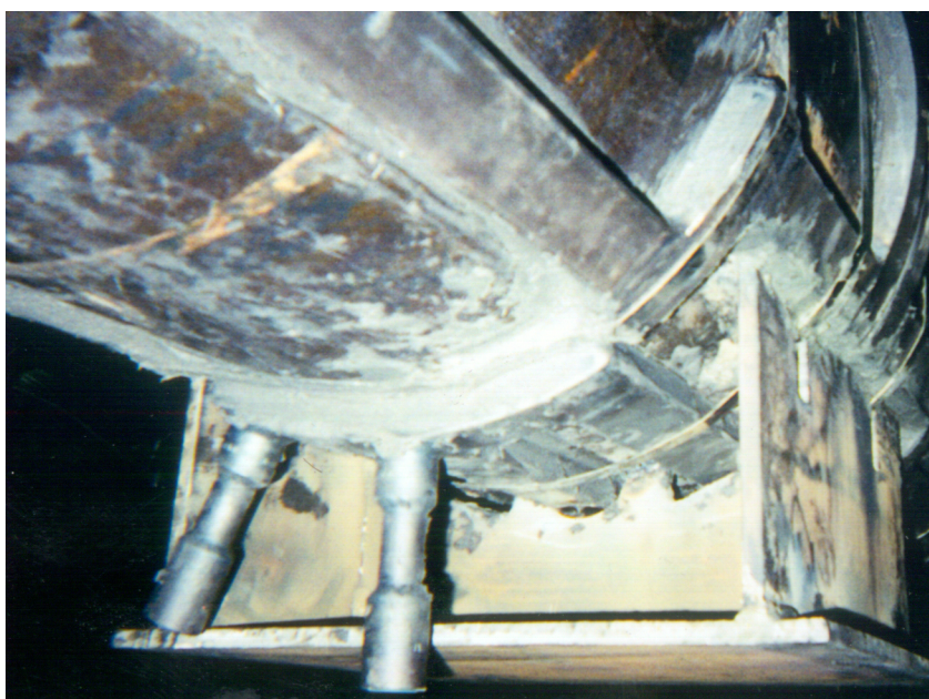
Fig 4: ControTrace at a pipe support.
