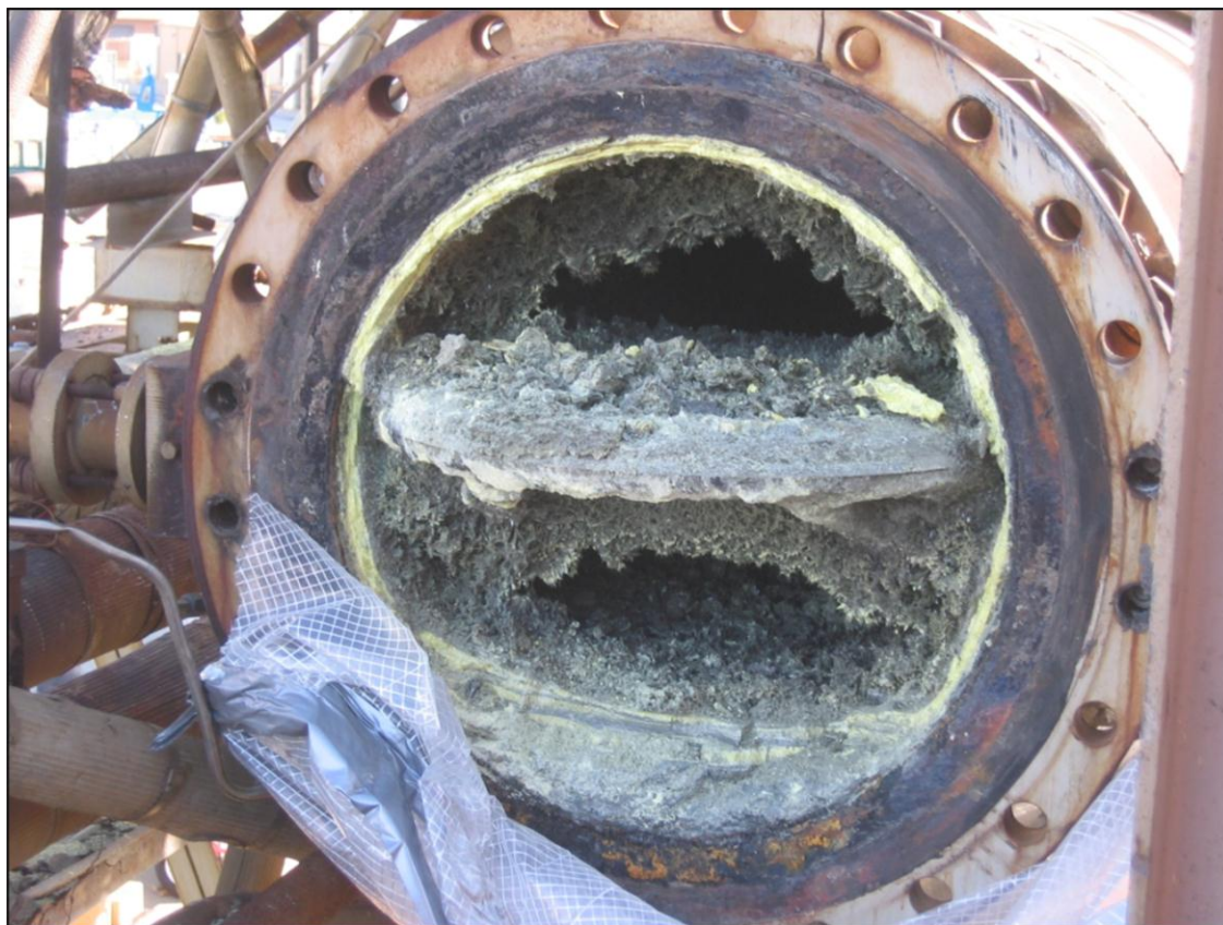
Figure 4: SRU Vapor Line Failure due to Plugging
