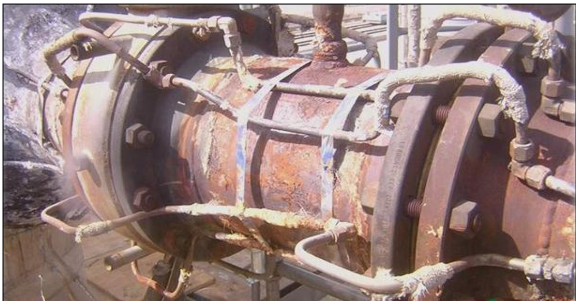
Figure 2: Convective Tube Tracing Installed on Large-Bore Piping
