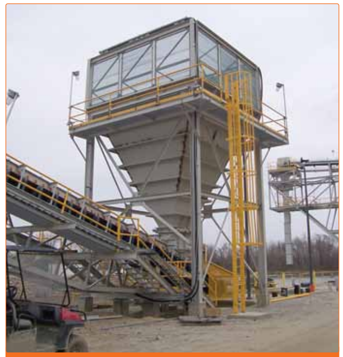
Figure 2. Fogging 'scrubs' the dusty air as material is discharged, as with this limestone hopper.
