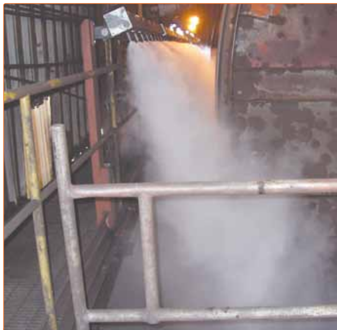
Figure 3. Installing dry fog systems, rather than dust collectors, requires less power and little maintenance.
